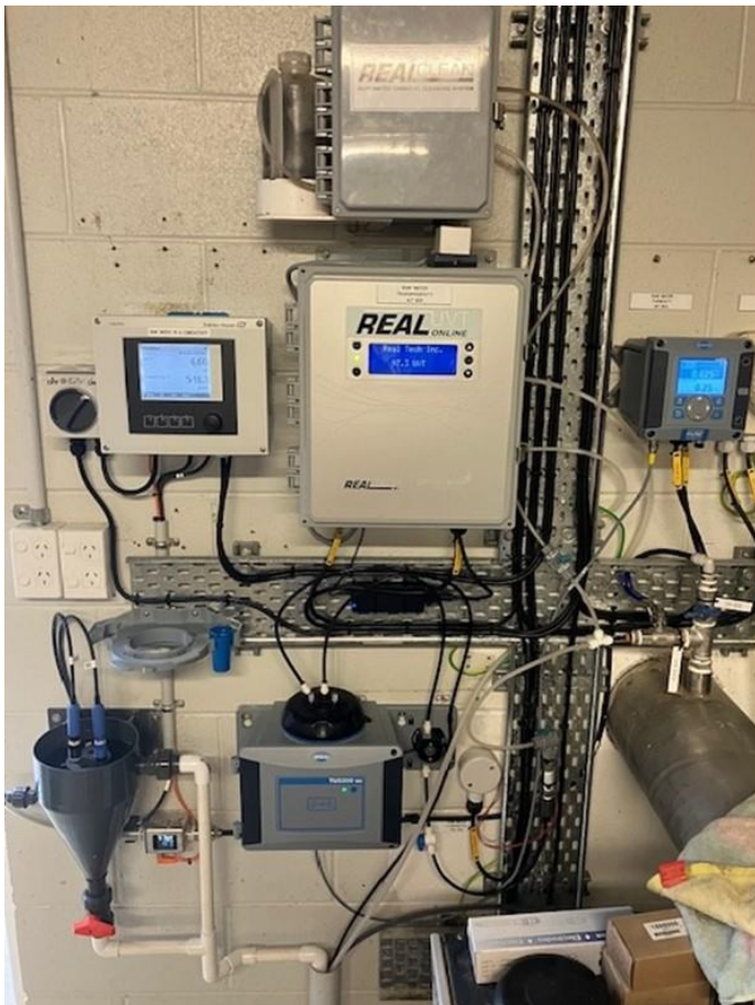
Treatment Plant - Turbidity, pH, conductivity, and UVT analysers
