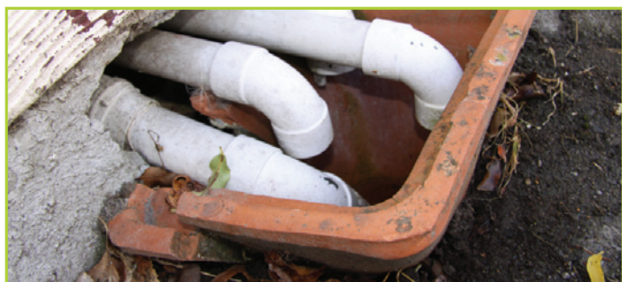
House waste pipes entering a damaged gully trap
