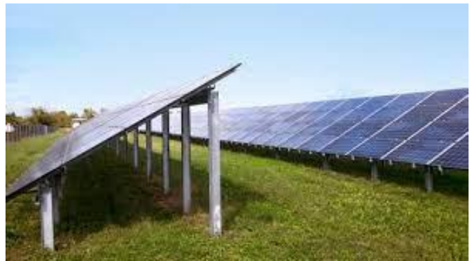
Fixed tilt solar farm
