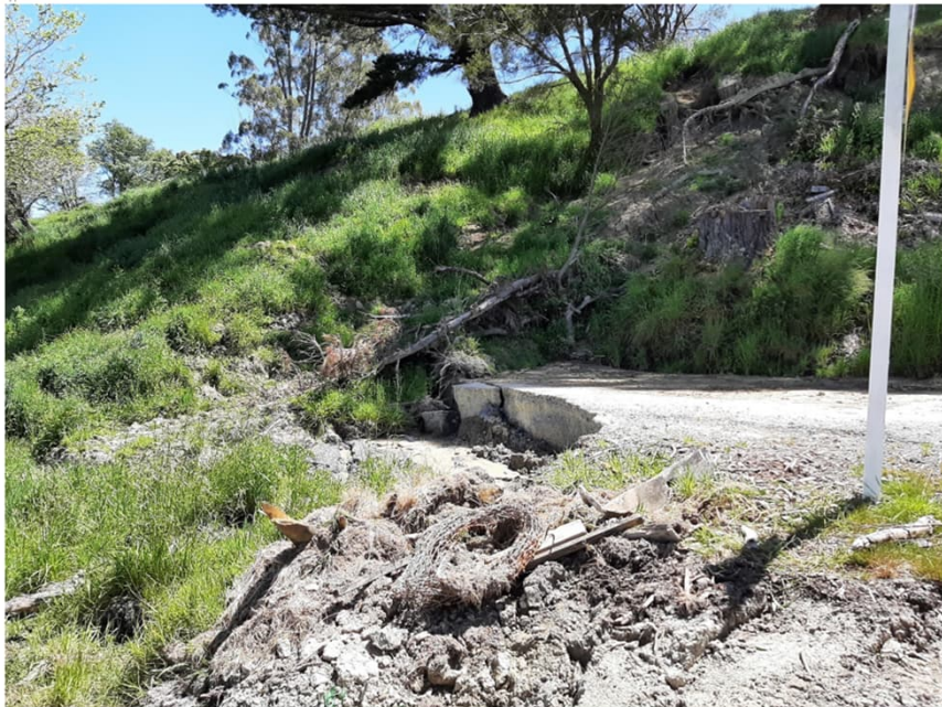
Photo 1: East end of landslide
