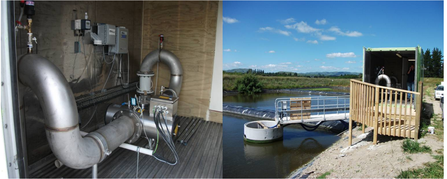
UV Reactor installed at the Martinborough wastewater plant
