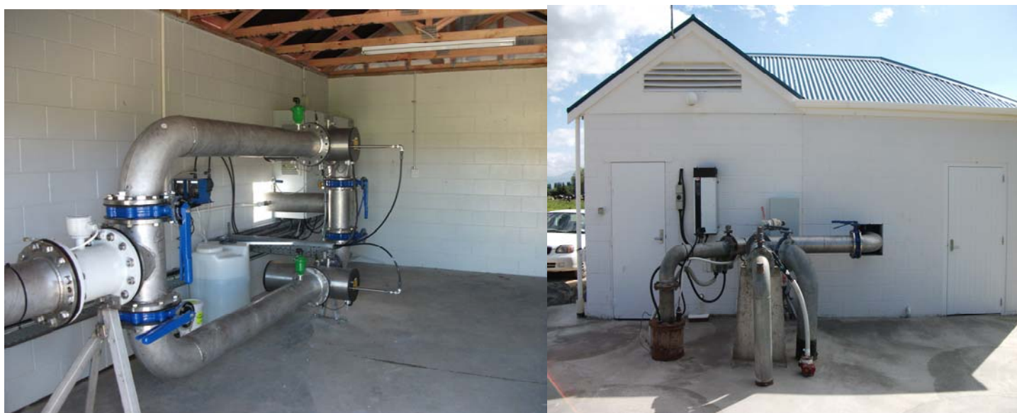
UV reactors installed at the Martinborough water supply bores
