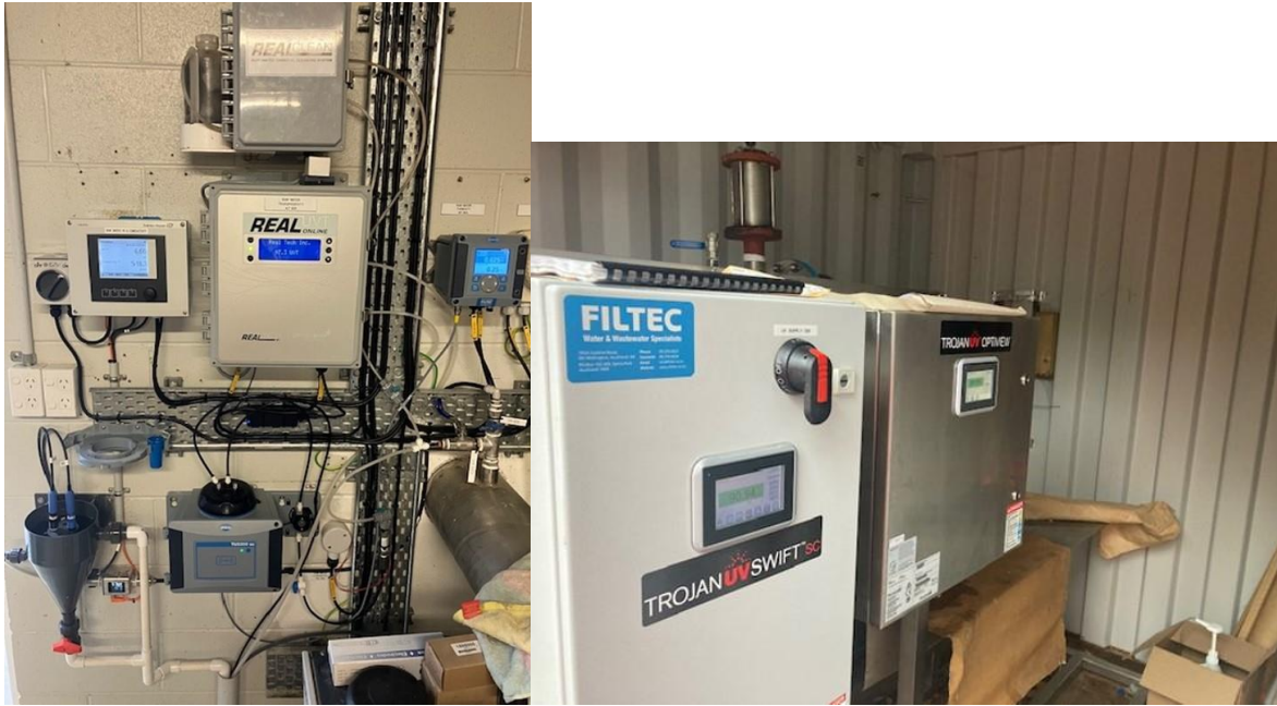
Treatment Plant - Turbidity, pH, conductivity, and UVT analyser
