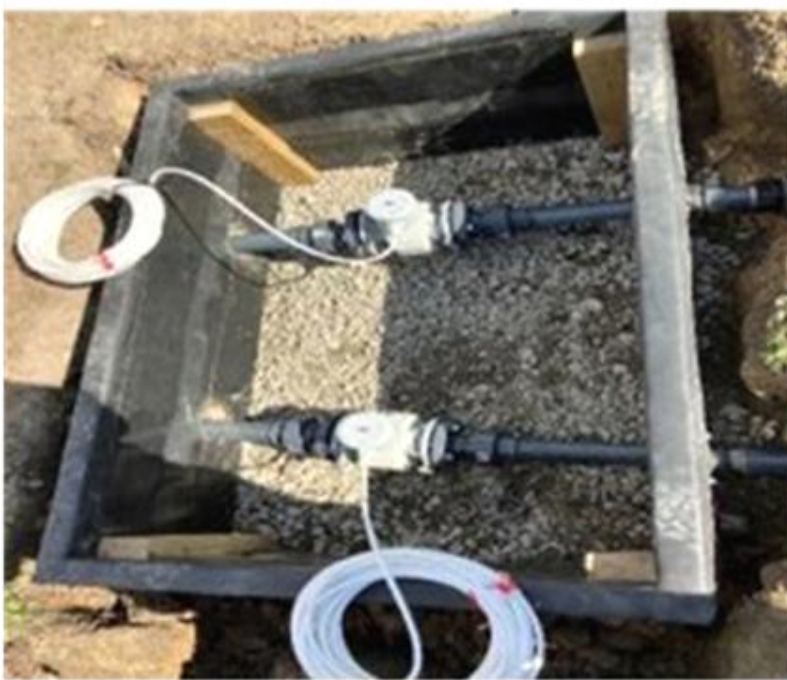
Photograph above: New flow meters that feed into the SCADA system
