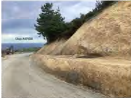
Example of retreating the road away from the under slip.
