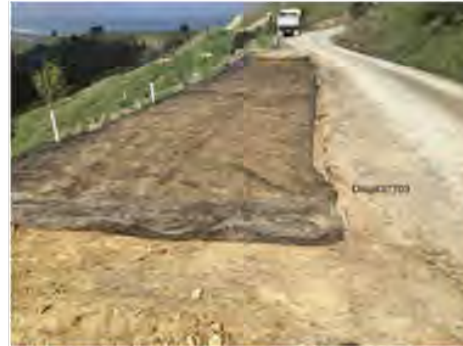
Example of a site where it was bench and reinstate the carriageway with reinforced fill
