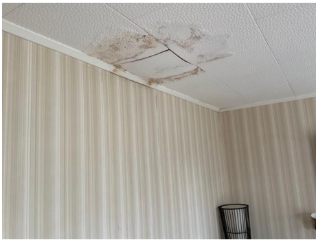
House - water damage
