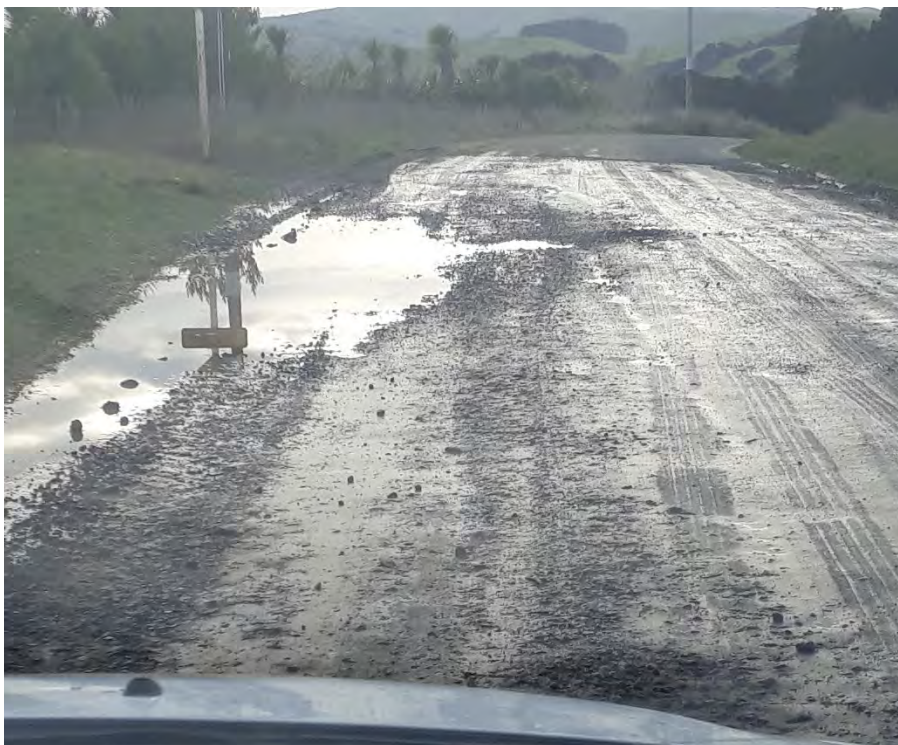
Figure 1 Safety Issue on corner
