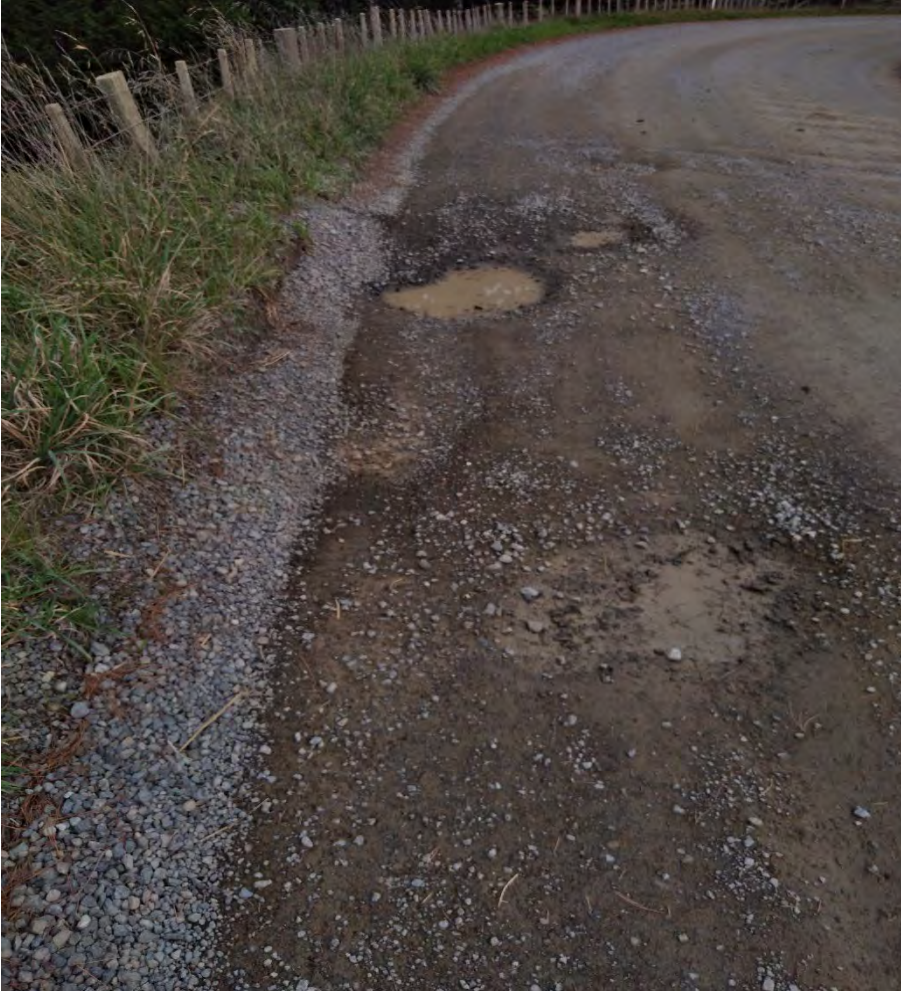
Figure 6 Potholes & corrugations - unsafe corner
