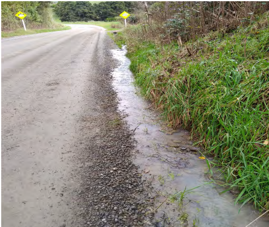
Figure 5 Vegetation obstructing drainage
