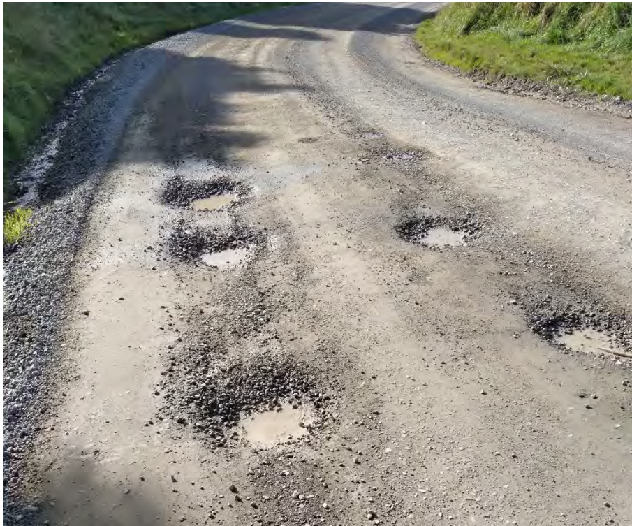
Figure 2 Safety on corner and Vehicle damage
