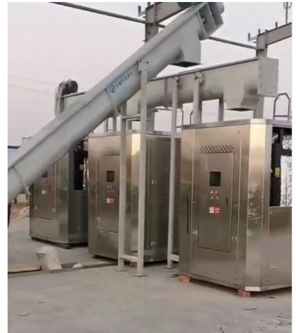
Multi-unit ROSIE's process 15t /batch
