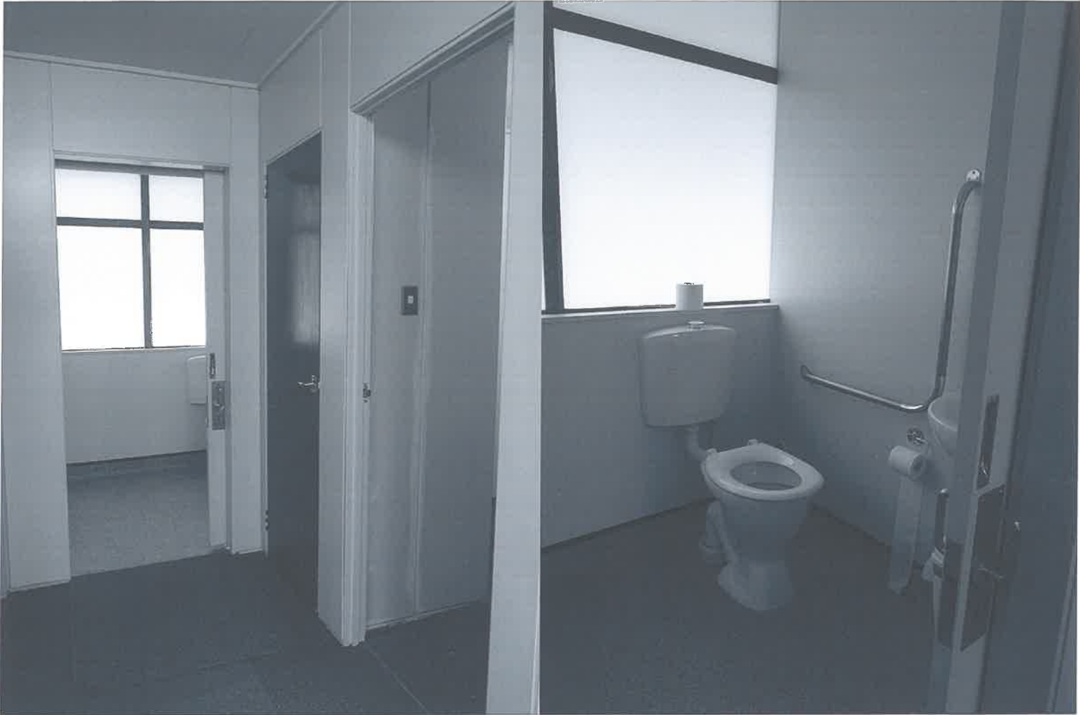
Examples of washroom and toilet upgrade, incl new disability toilet and fire exists upgrades, Featherston Community Centre, 2014.
