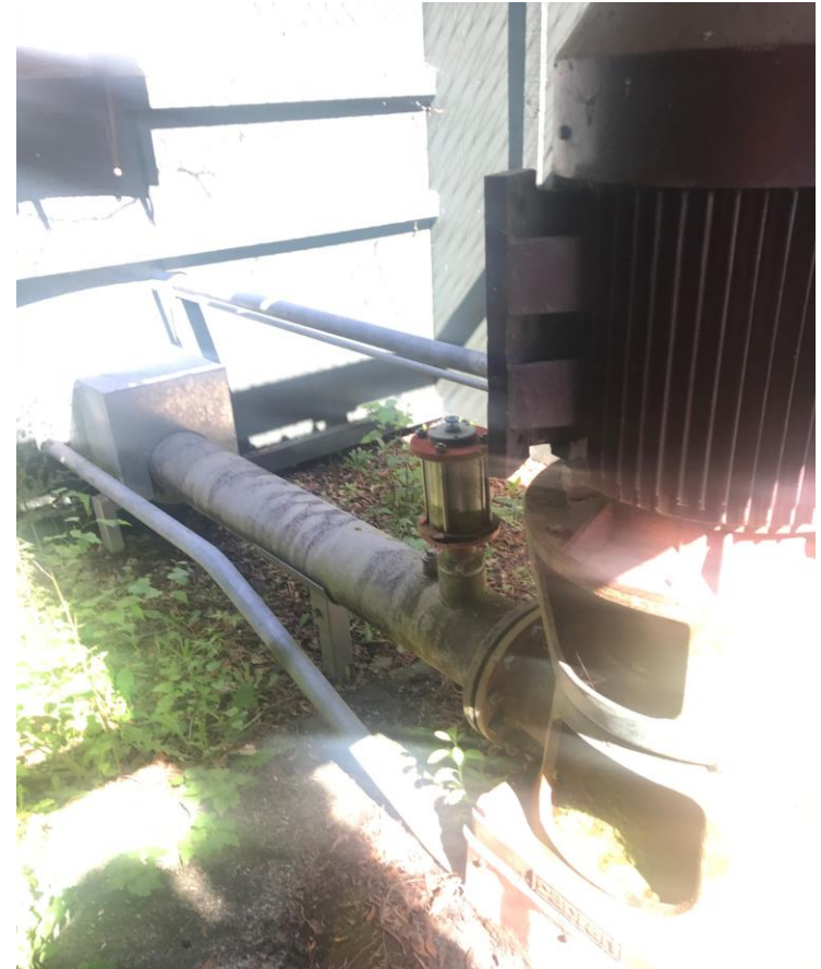
The existing bore pump at Memorial Park
