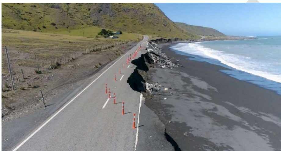
Figure 3 Exposed part of the Cape Palliser / Mātakitaki-a-Kupe Road
