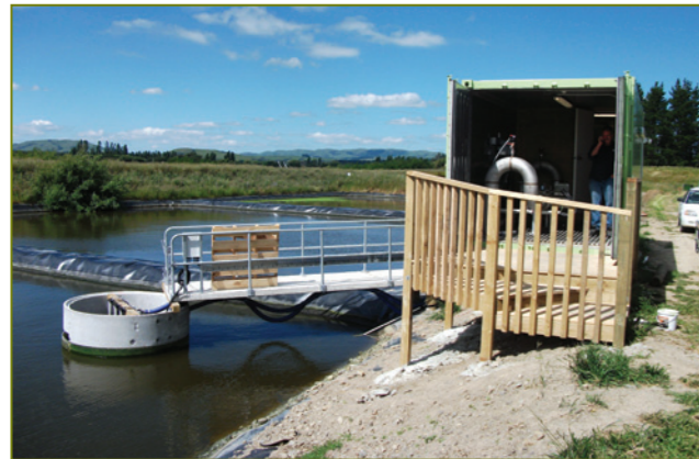
The image shows the new plant in its housing adjacent to the maturation cells at the wastewater treatment plant
