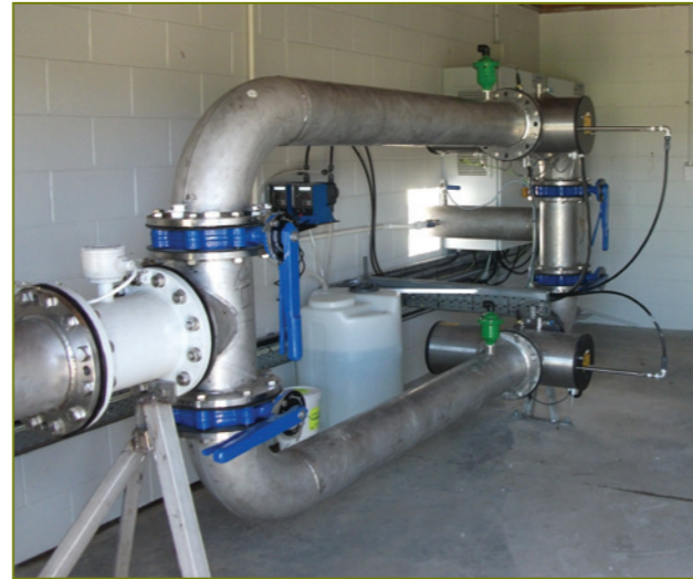
The image shows the two UV units that have been placed within a new extension to the plant building at the Herricks bore site
