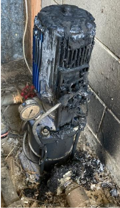
Figure 1. Burnt-out water pump, Martinborough
