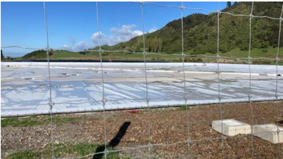
Figure 5. Photo of filled treated water reservoir bladder at Waiohine WTP
