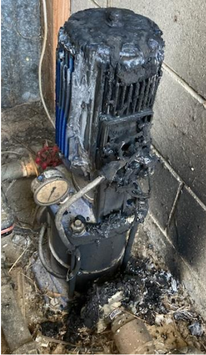
Figure 1. Burnt-out water pump, Martinborough
