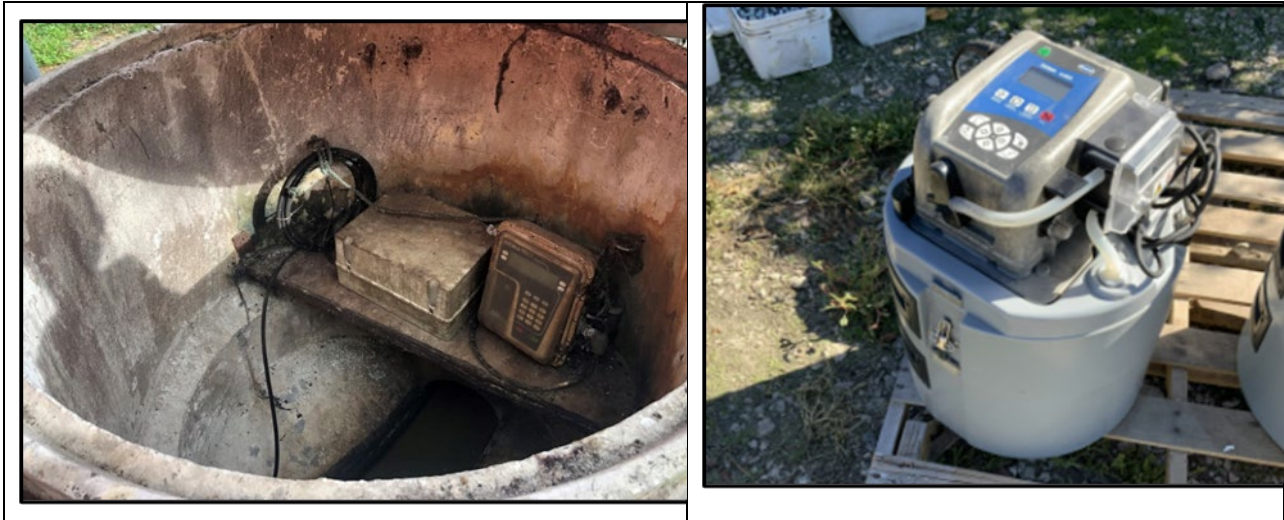
Figure 3 - MWWTP influent flowmeter (left) and typical portable composite sampler (right).
