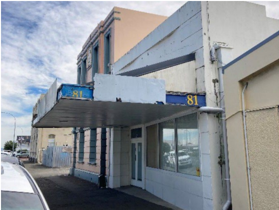
Deteriorating building. Childers Rd
