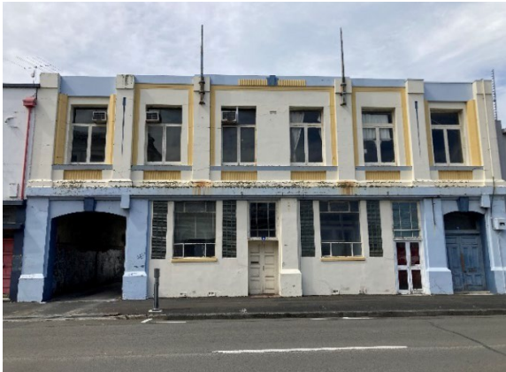
Deteriorating building. Lowe St
