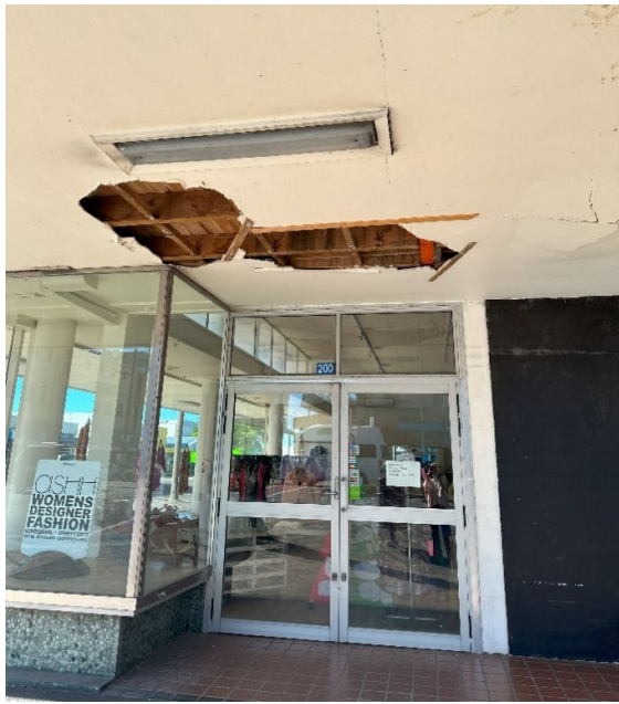
Main Street building decay. Gladstone Rd
