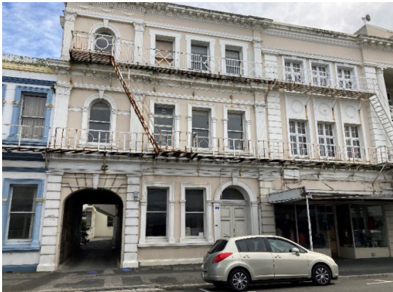
Masonic Hotel decaying façade. Lowe St
