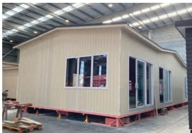
Progress photos show the build in situ at the Presidential Homes facility in Palmerston North where the construction takes place in a large warehouse.
