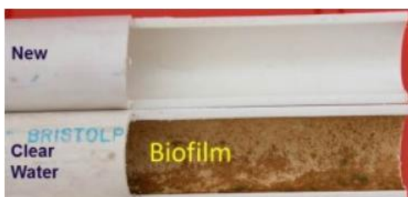
Image 3 – Biofilm inside a pipe
