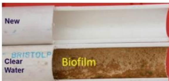
Image 3 – Biofilm inside a pipe
