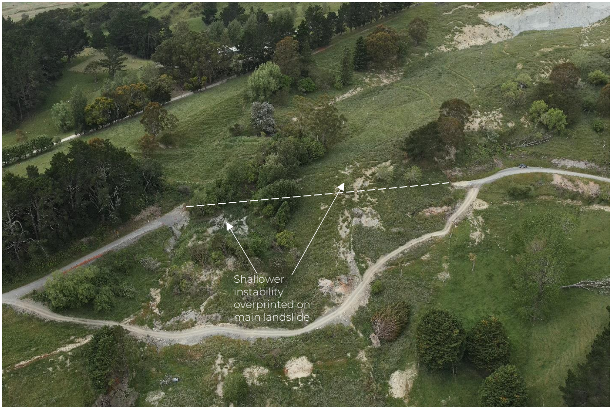
Figure 4: Site as at 14 December 2022, with lower 4WD track in foreground constructed on 'rafts' of pavement displaced downslope from Hinekura Road (approx. original road dashed).
