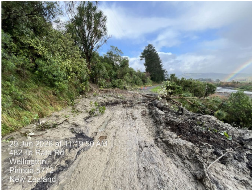
Figure 8: Deris from upslope deposited on road carriageway
