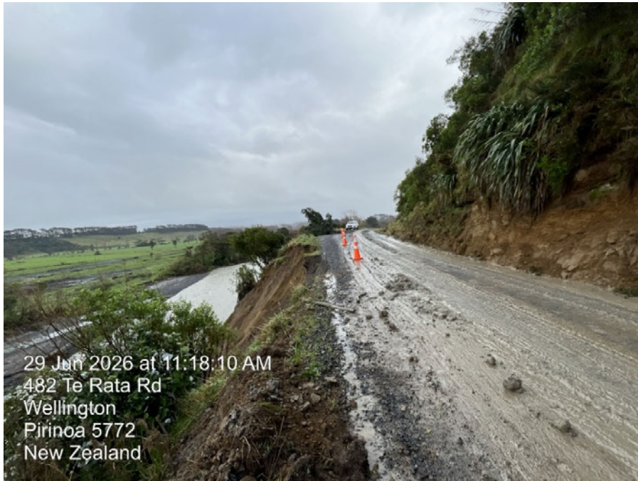
Figure 6: Road shoulder has been lost due to under-slip (Looking Southwest)
