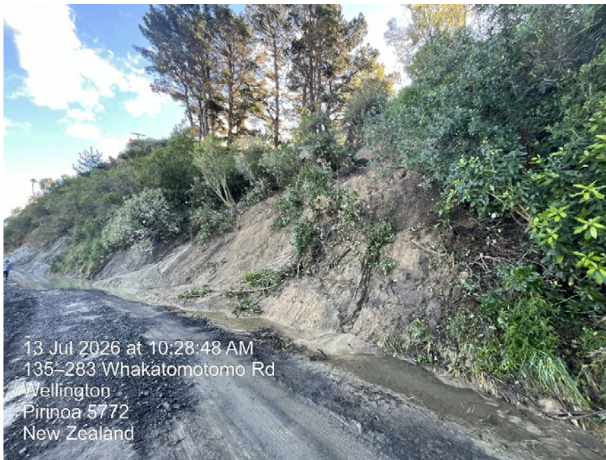
Figure 9: Debris from the upslope blocking the swale and culvert inlet, causing ponding and stagnant water on the road surface
