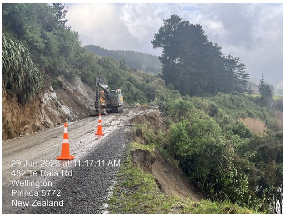
Figure 5: Road shoulder has been lost due to under-slip (Looking Southeast)
