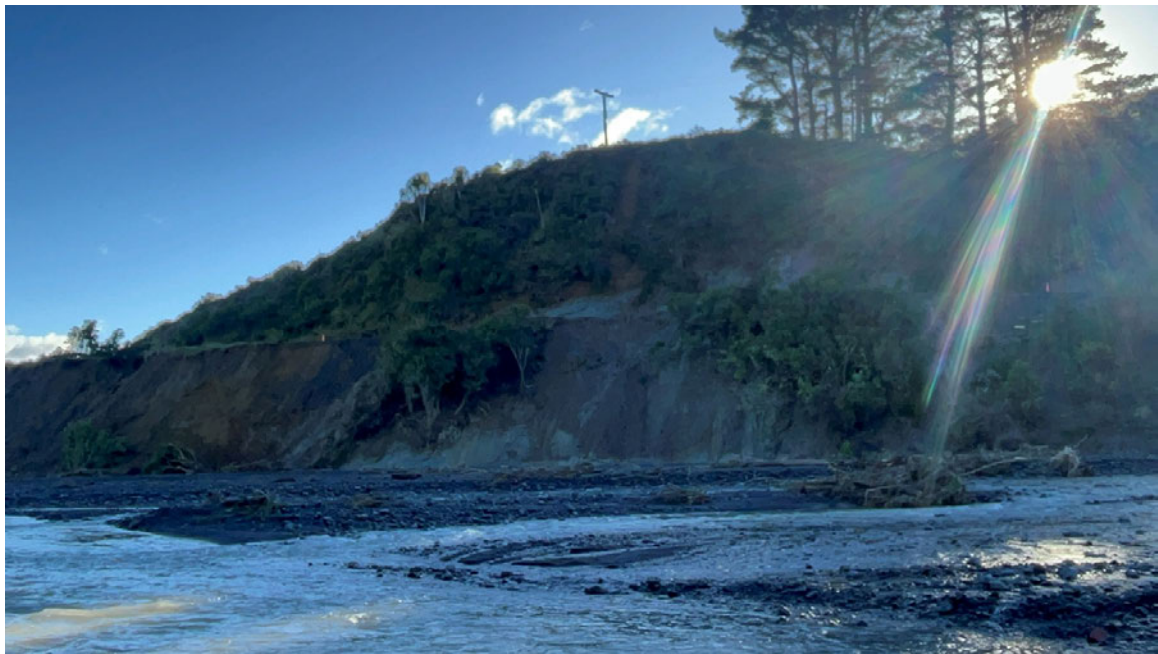
Figure 4: Landslide on both upslope and downslope at Whakatomotomo Road RP 2.650 to RP 2.850 (view from Te Rata Road)
