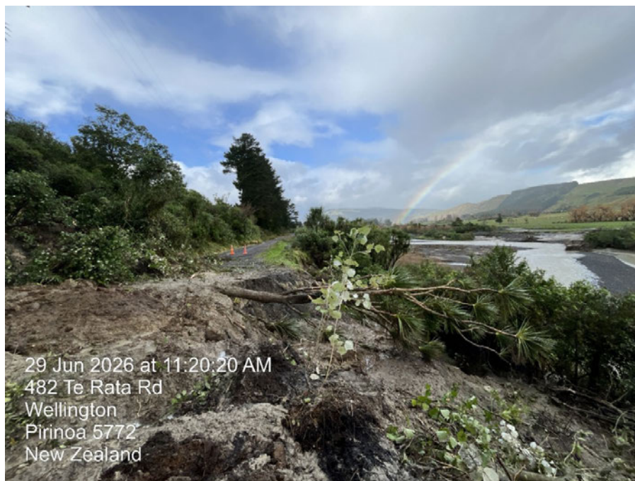
Figure 11: Road carriageway has been lost approximately 1m due to under-slip
