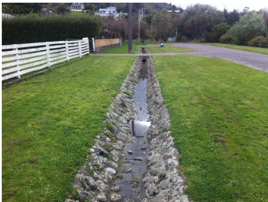
Figure 29 Lined storm water drain
